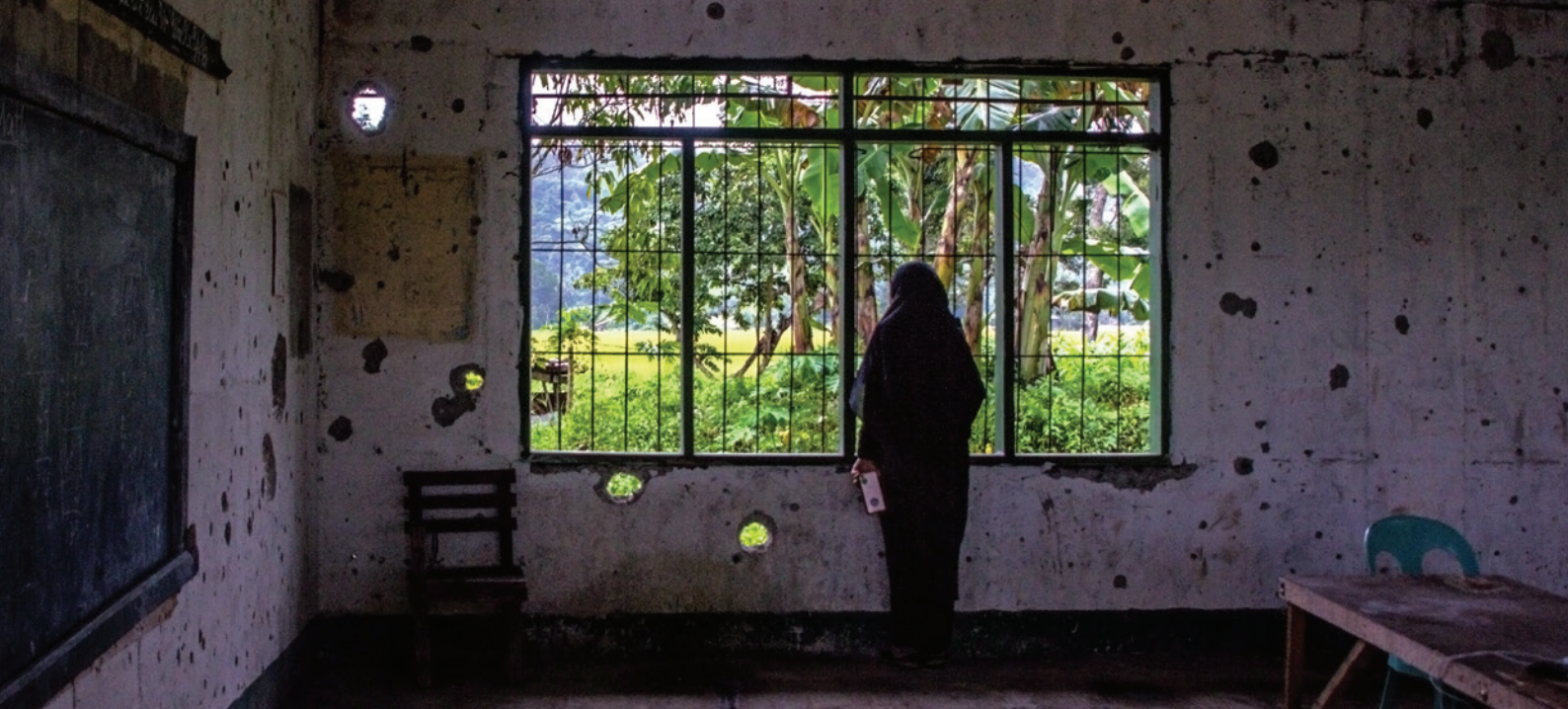
A bullet-riddled classroom in Ranao Elementary School, Butig, Lanao del Sur. The school was badly damaged during the 2016 armed clashes between Dawlah Islamiya (DI) and the military. Barangay Ragayan is located next to Barangay Poctan, where the main training camp of DI was situated. 📍 Najib Zacaria
